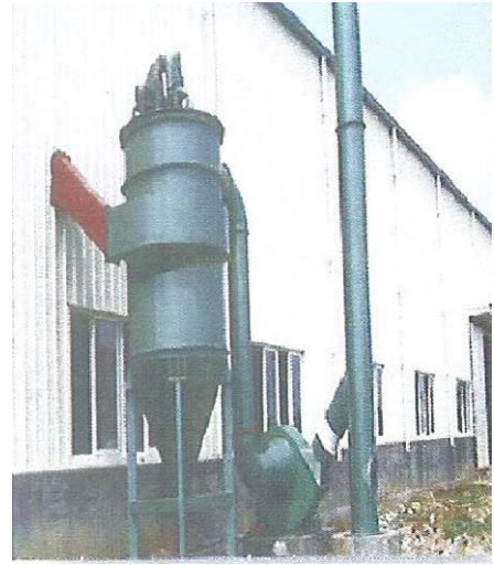
Figure 3 Dust collector system.
